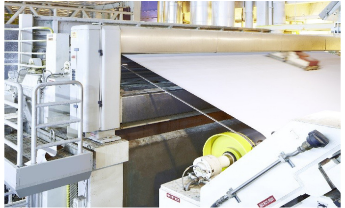
04 The mill uses ABB Quality Control Systems. Pictured here is an ABB Network Platform that is scanning the paper web to ensure that all quality parameters are met.
