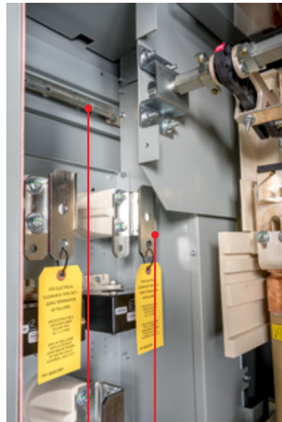
Ground bus link
