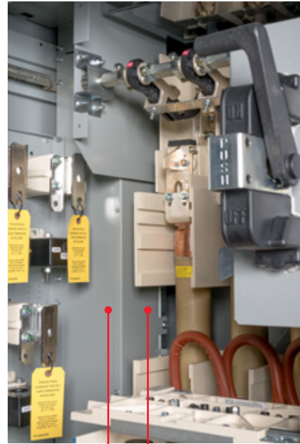
Motor cable trough barriers
