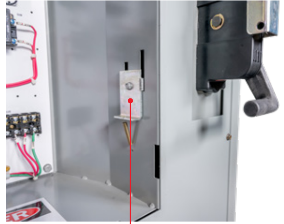
Door interlock defeater
