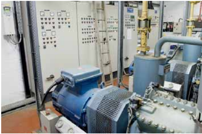
Drives are installed in condenser fans, air compressors and water pumps.
