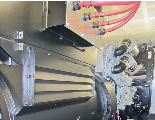
Emergency generator set supplying 2,000 kVA / 11 kV
