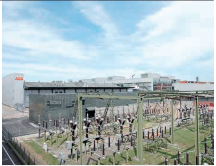
5b The ABB HV GIS factory can be seen behind the substation.
