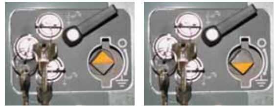
Earthing switch open.
