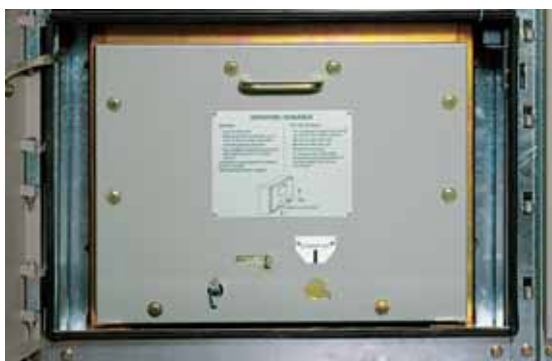
VT compartment with withdrawable voltage transformers.
