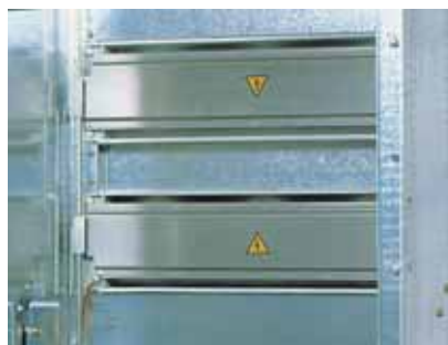
Metal segregation shutters.
