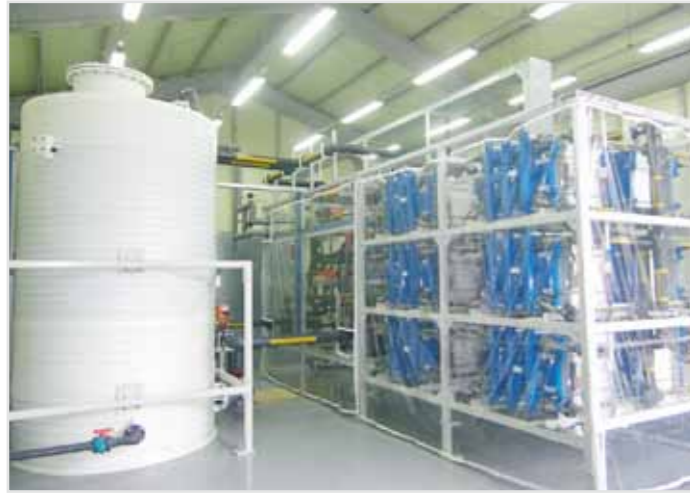
ABB's PCS100 ESS and Prudent's VRB Energy Storage System that has been installed on Jeju Island located in between Korea and Japan
