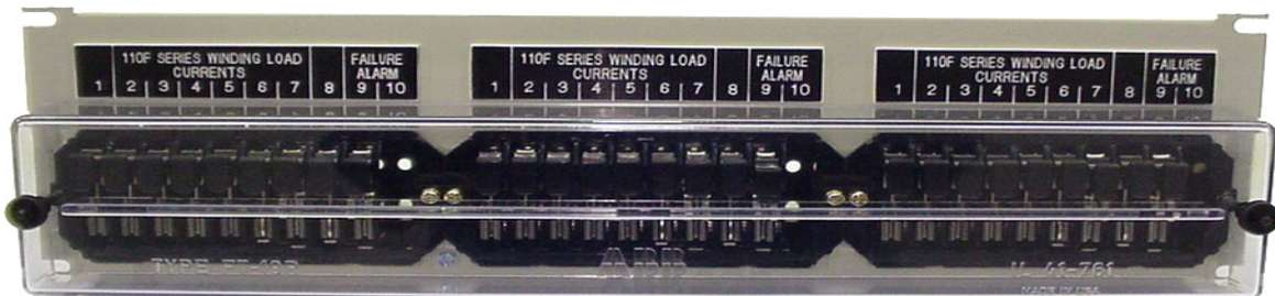
FT-19 3RU with Full Length Clear Cover. Switches mounted in the lower position, with special customer labels
