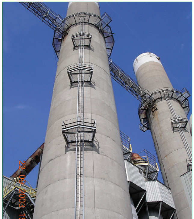
Location of the sample extraction equipment on the stack.
