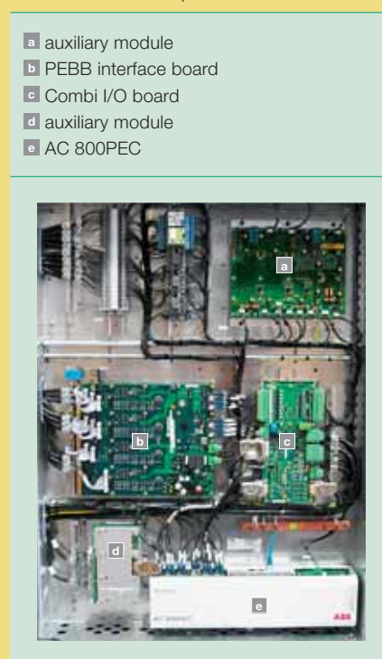
3 Control hardware panel of CC750®
