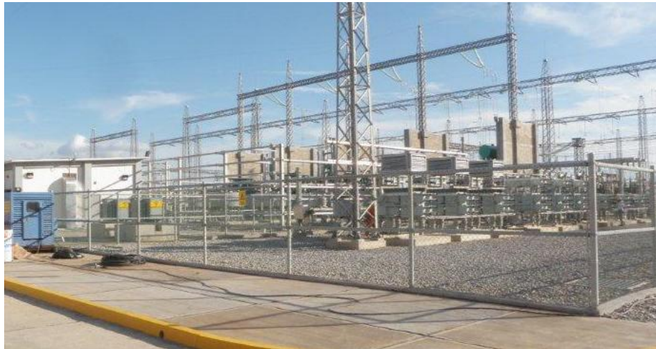
Fig. 6: 400 kV SVC at La Ventosa, Mexico
