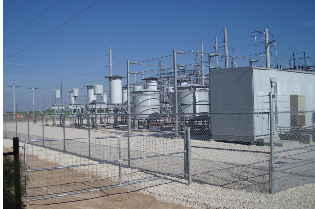
Fig. 5: Crane 69kV, -40/+50 Mvar SVC
