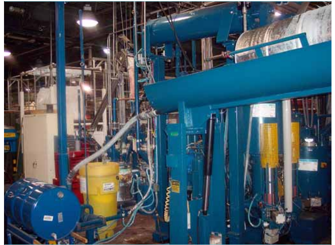
6 Epoxy blending equipment in ABB's Pinetops facility in North Carolina.
