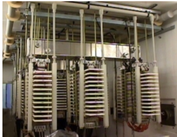
Fig. 11: SVC Light valve
