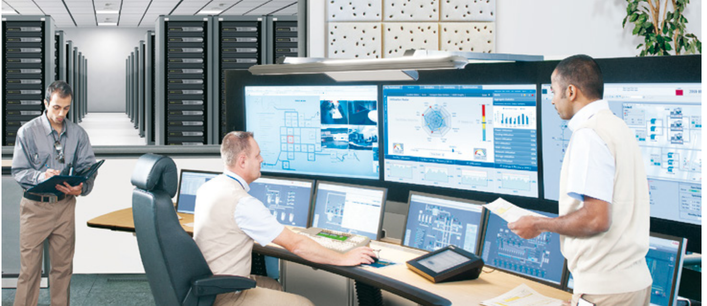
Decathlon Data Center Enterprise Management – enabling predictive reliability and energy efficiency for today's data centers.
