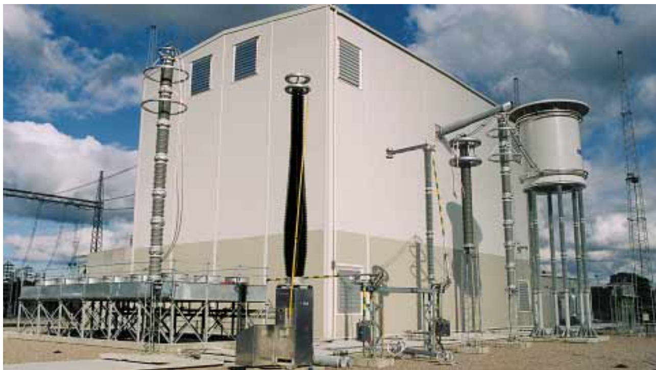
3 Valve building in the Slupsk (Poland) converter station
