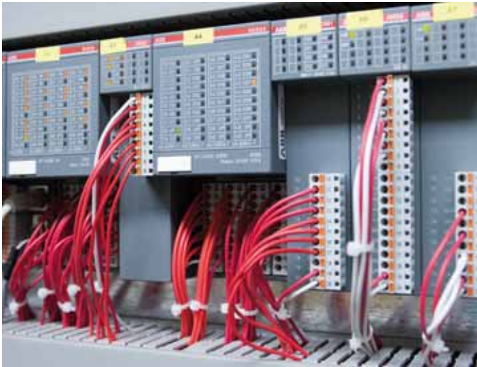
Temperature control in the extrusion process is critical. It requires precise calculations, so ABB developed a temperature control program for the PLCs used by Sarem.
