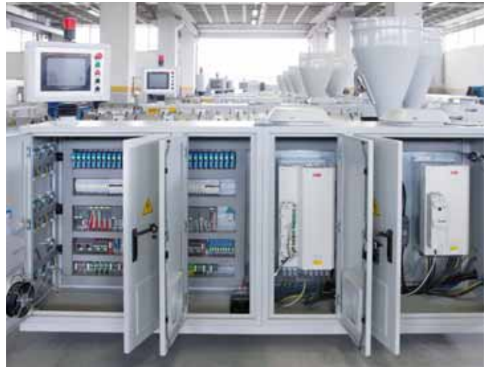
Sarem installs ABB's drives, motors, operator panels, PLCs and low voltage products in their machines.
