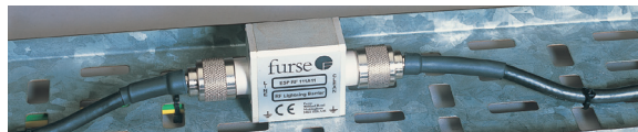
Figure 4: ESP RF 111A11 installed on a coaxial cable running between an antenna and a RF receiver. Note the earth lead (behind the cable tray) attached to the mounting fixture.
