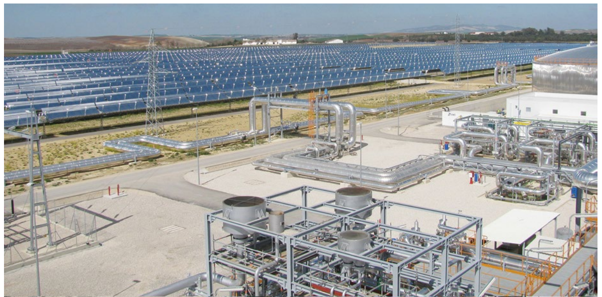
Aerial view of one of the storage systems and the power blocks at Valle 1 and Valle 2 solar thermal power plants. (© SENER / TORRESOL ENERGY)
