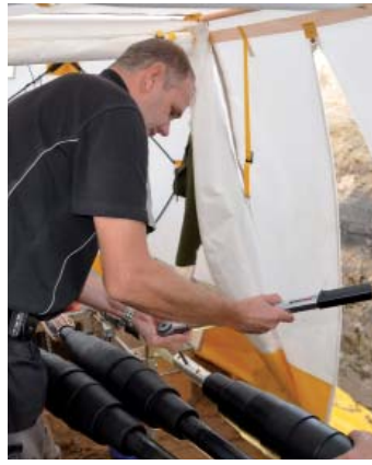
JS-A 72 kV installation.
