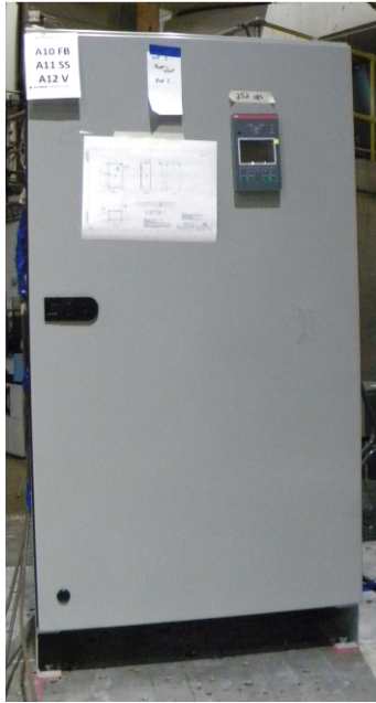
Floor Mounted UUTs
