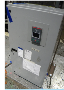
Wall Mounted UUTs
