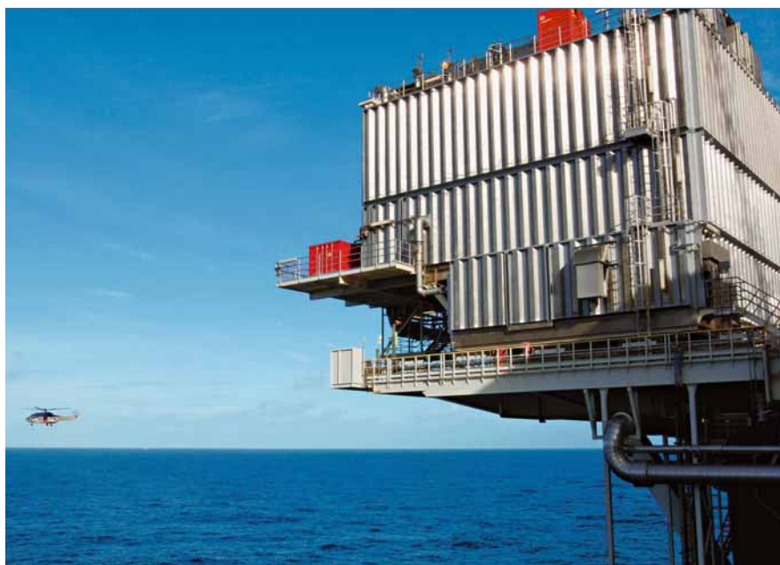
2 HVDC Light module on Statoil's Troll-A platform
