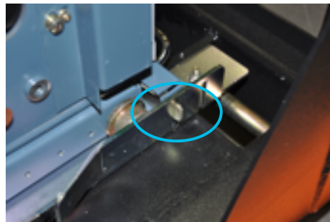
Figure 5-5. SecoVac VCB Tab Locked in Lift Truck Slot
