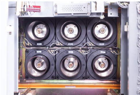
Figure 9-2: CTs Mounted in Compartment
