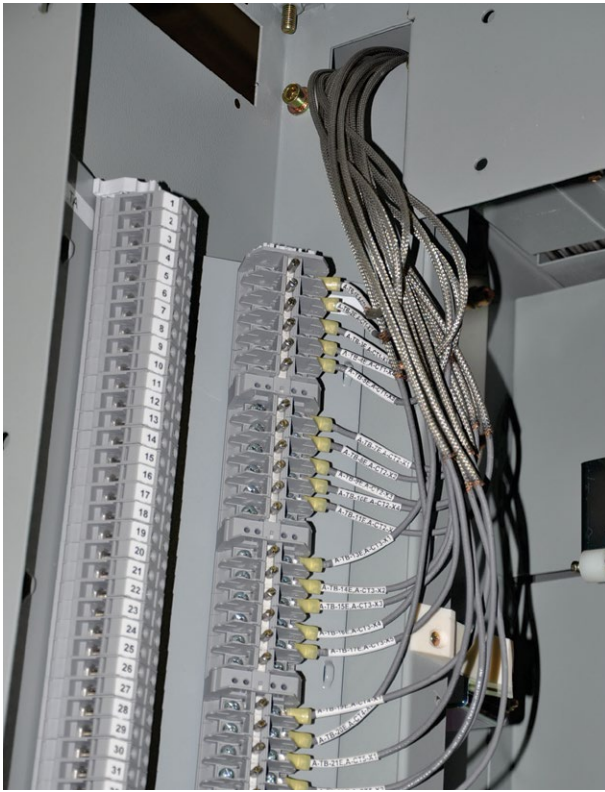
Figure 9-6: Shorting Terminal Blocks
