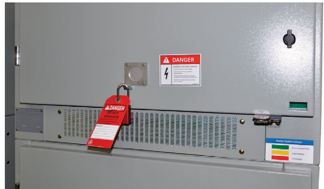
Figure 9-8: SecoGear Manual Racking Port Padlocked
