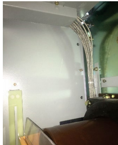
Figure 9-5: CT Wire Harness in Compartment
