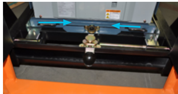
Figure 5-17. Unlock VCB from Lift Truck
