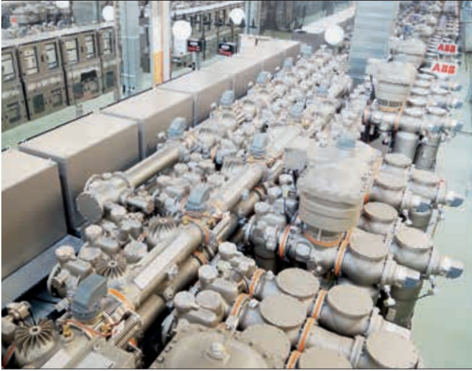
3a GIS AT 170 kV
