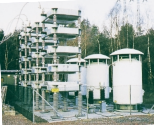
Prototype ConTune AC filter in the Lindome terminal of the Konti-Skan HVDC link 5
