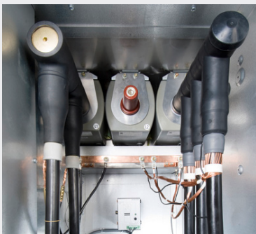
Cable compartment with current transformers
