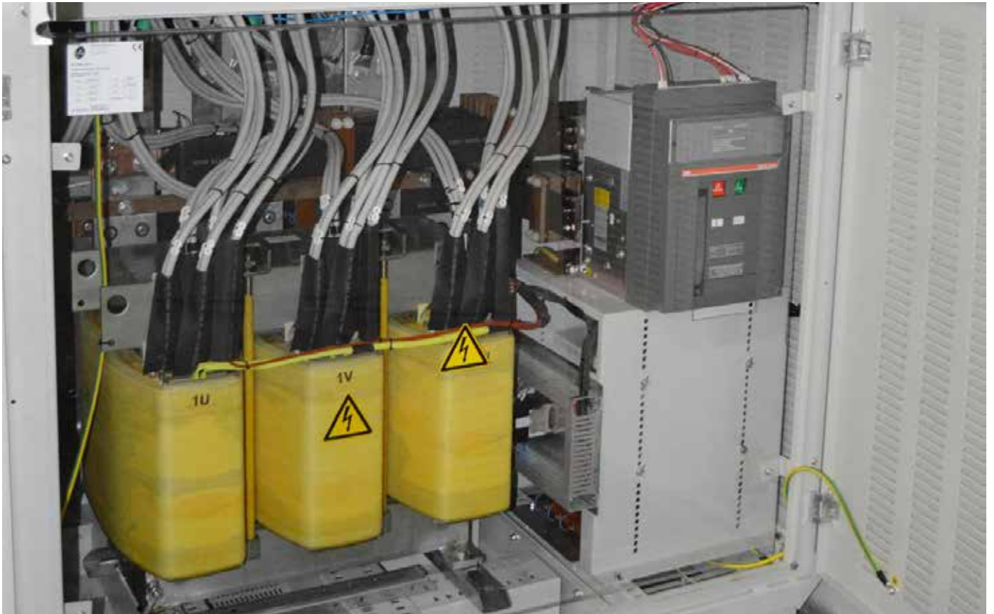
Emax by ABB SACE division installed inside E-Power
