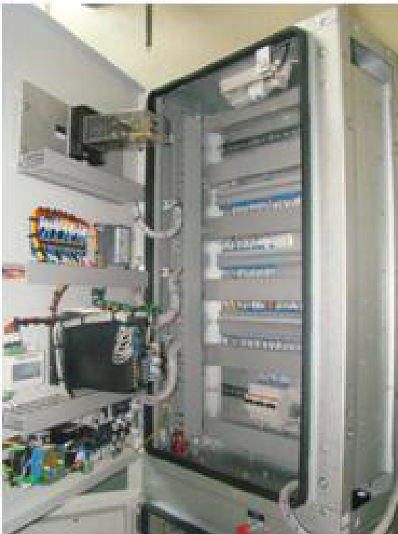
Fig.41 Low Voltage compartment
