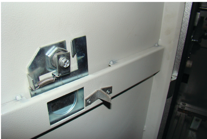
Fig.16 Circuit-breaker compartment door enabling device
