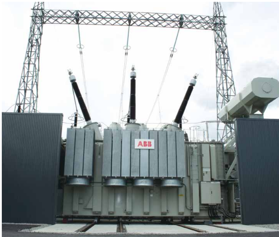
HVDC transformer at Songo
