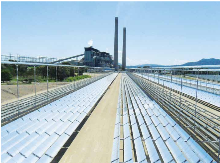
World's first solar hybrid coal-fired power station of ABB in Liddell, Australia
