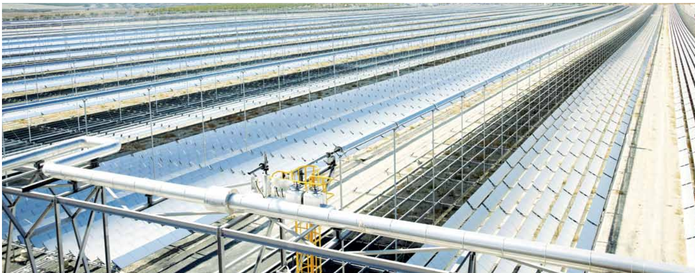
Novatec Solar technology holds the key to renewable energy development
