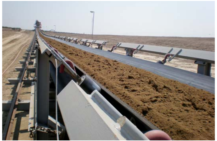
15,000 rollers support the conveyor belts.
