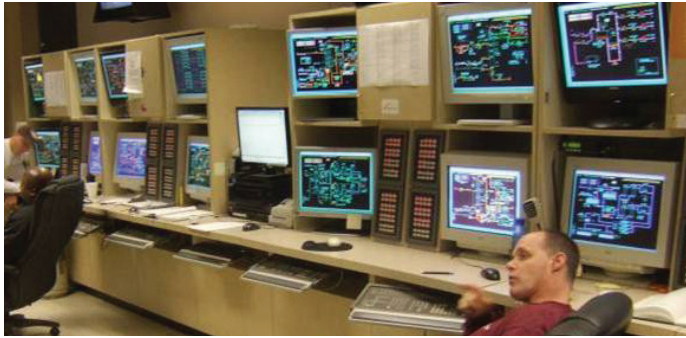
Control room at Arkema Inc., Calvert City plant
