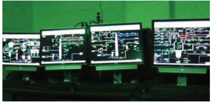
ABB System 800xA workstations in staging
