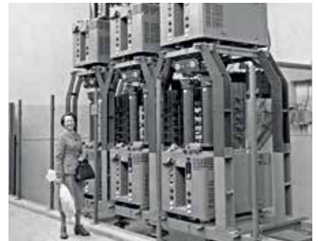
1954 First commercial HVDC transmission line connecting Gotland island with the Swedish mainland (ASEA)
