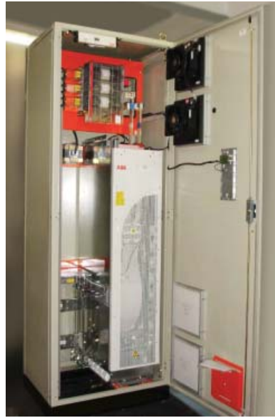
The ABB industrial drives control the furnace air flow by adjusting the speed of the fan motors.
