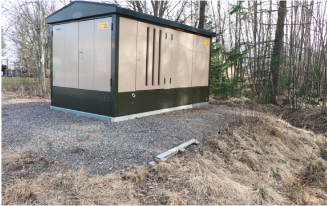
Prefabricated substation on the small hill with proper ground preparation ...
