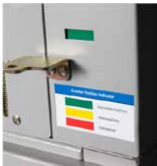
Figure 6-3: Breaker Position – Disconnect (Green)
