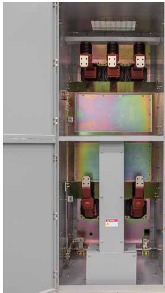
Figure 6-20: Rear View of Two high Compartment Showing Cable Trough
