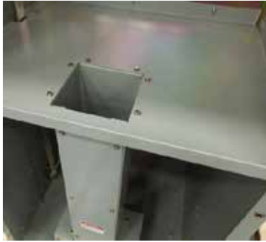
Figure 6-21: Cable Trough Opening
