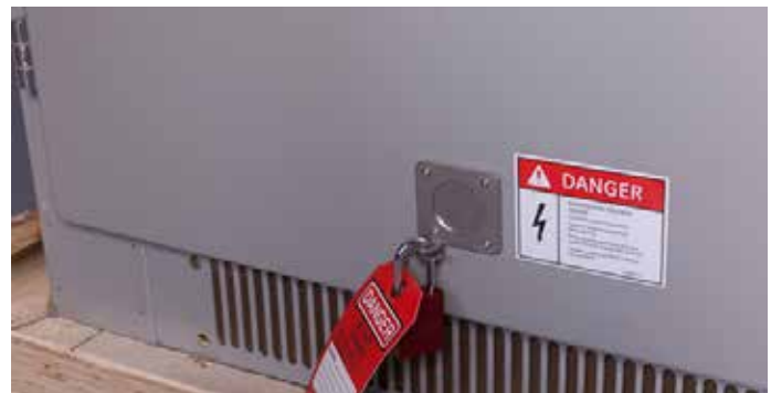
Figure 6-13: Breaker Racking Padlock
