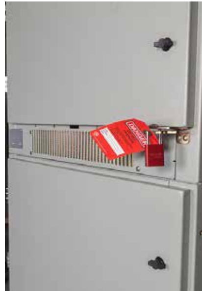
Figure 6-12: Front Door Padlocking Provision
