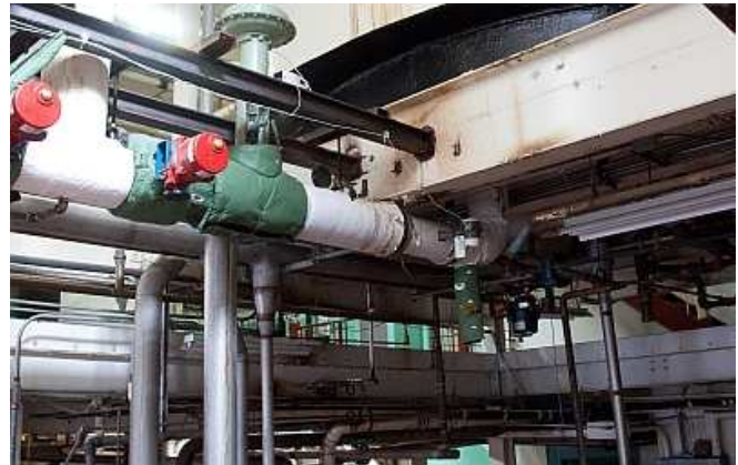
Figure 2. Tight piping geometry led to the choice of Swirl meters, which have minimum straight pipe requirements.
