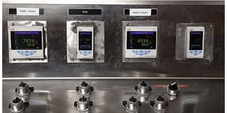
Figure 4. Panel containing ABB CM30s and CM 10s.
