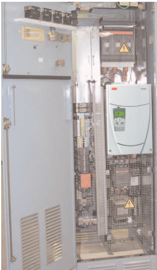
DCS800-E mounted in old cabinet
