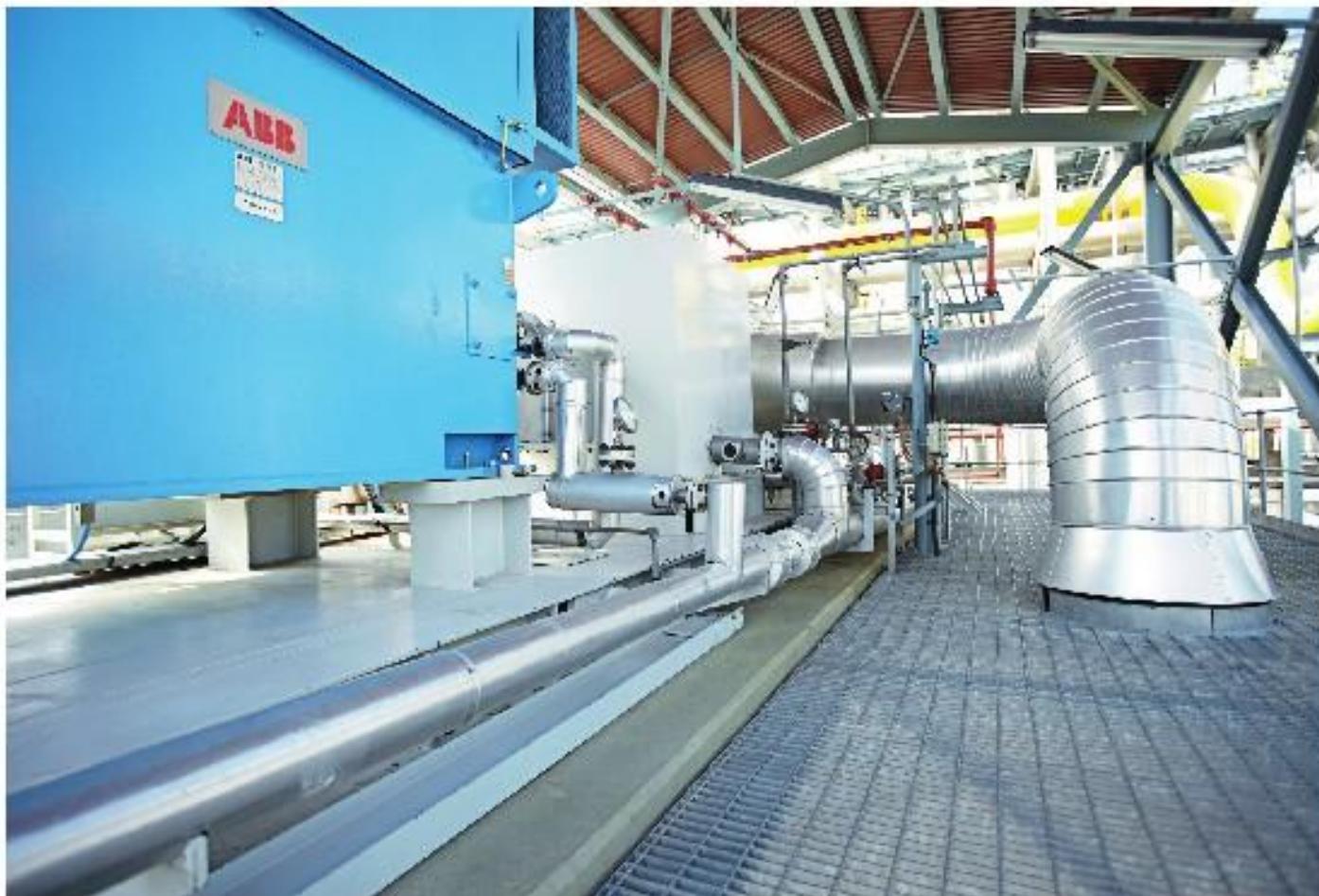
ABB is introducing a new line of gas compression modules designed for relentless and efficient operation.
