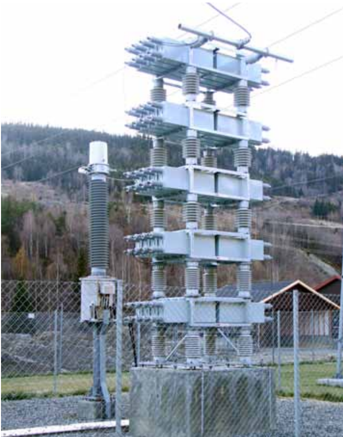
Vågåmo 100 Mvar shunt capacitor bank installed and commissioned in 2007
