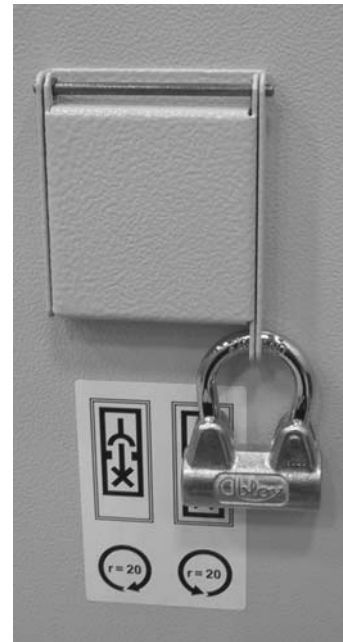
Figure 3.13 Using the padlock (withdrawable type cubicle).
