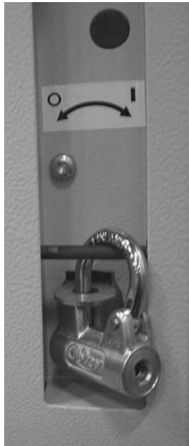
Figure 3.12 Using the padlock (withdrawable type cubicle).
