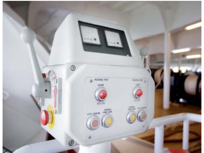
Winch operator controls were easily integrated with the drive's I/O.
