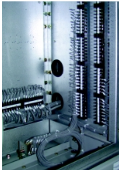
38-inch instrument compartment with TOC switch and terminal blocks for customer wiring and interframe connections.
