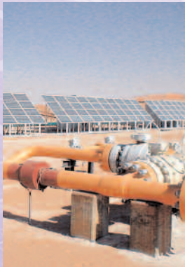
Photovoltaic system at an industrial site
