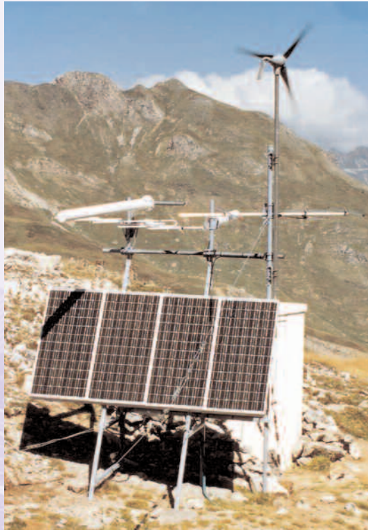
Standalone system at the Pourtalet pass, France
