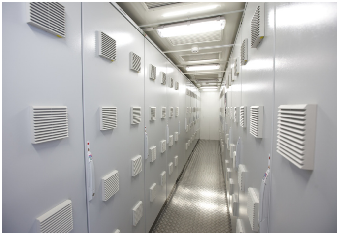
Battery container with LG Chem battery
