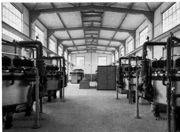
Fig. 3. — Mutator plant for an aluminium works; four double sets of, each, 11,000 A, 600 V, total 26,400 kW.
