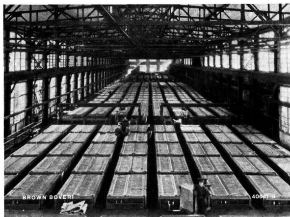
Fig. 2. — Electrolytic cell room in a zinc works supplied by grid-controlled mutators 30,000 A, 460–560 V.
