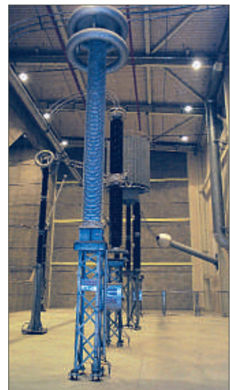
3 Indoor DC yard at Zhengping converter station (3GC)
