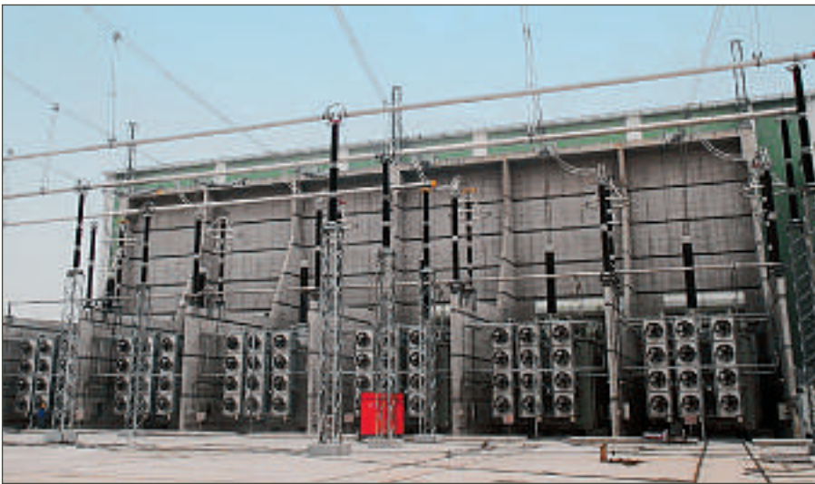
7 Converter transformer arrangement per pole
