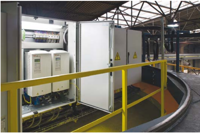
ABB industrial drives bring accurate control when lifting aluminium plates.
