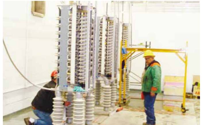
Fig. 2: State of the art ABB thyristor valve, replacing the much larger original valve from 1980.
