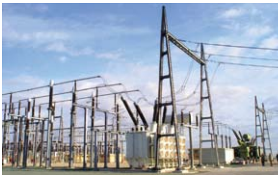
Spare Polytransformer in parallel operation with a 450 MVA unit, 400 kV.
