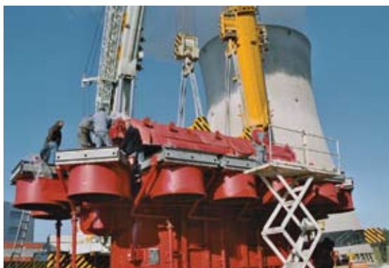
ABB's full service package ensures complete customer support and service.
