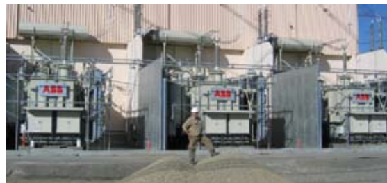
The world's largest HVDC transformers are installed at Sylmar East converter station, U.S.A. 620 MVA, 230 kV, single phase.
