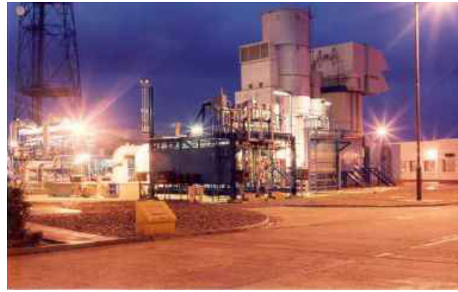
— Centrica Easington onshore terminal.
