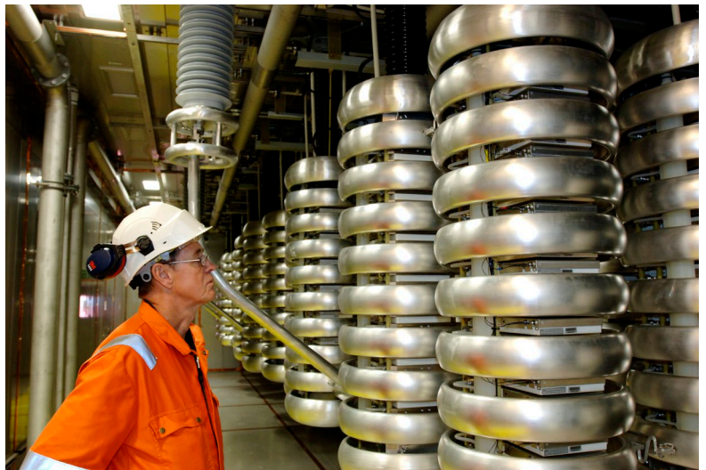
Figure 45: converters in an HVDC station
